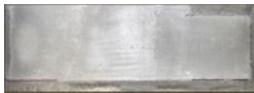
Mortar with good crack behavior.
